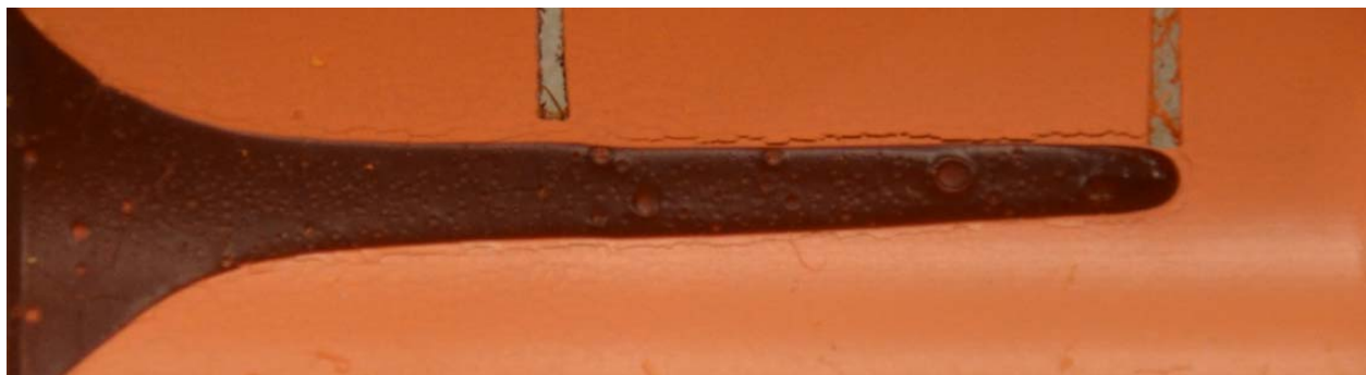
Figure 4. Cement dribble on inside of CPVC pipe with ESC cracks found around the periphery of the dribble.
